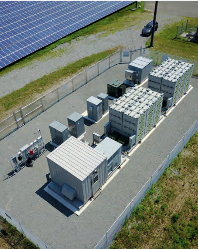
Photo: Eos Energy Storage
